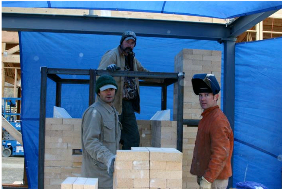
Founder and Executive Director David Hiltner building soda kiln with Matt Long and Frank Saliani.
